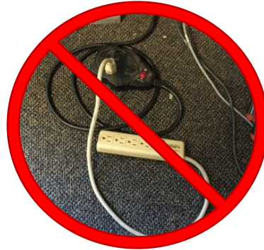
Photograph 2 –Surge Protector Energizing another Surge Protector
