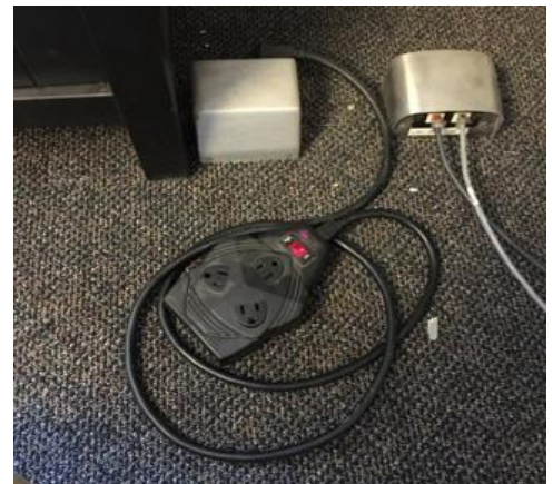
Photograph 1 – Surge Protected Multi-Plug Power Strip
