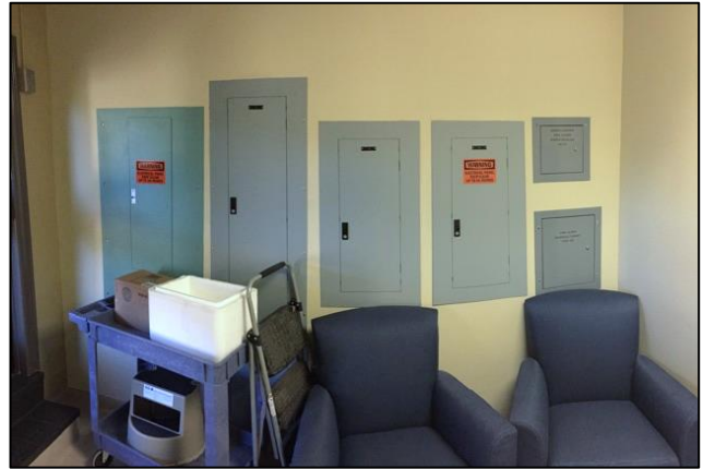
Photograph 1 – Blocked Electrical Equipment
